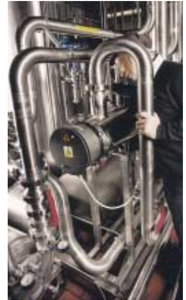
One million litres of water per day for soft drinks production is treated by Hanovia UV systems at the Silver Spring Mineral Water Company, England.
