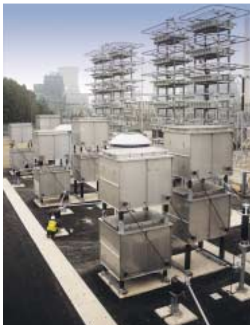
Cressall filter resistors improve power transmission efficiency at the Willington Power Station, England.
