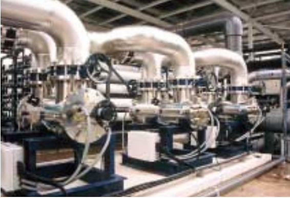
This Hanovia UV treatment plant at Bedok, Singapore, disinfects wastewater for reuse in irrigation.
